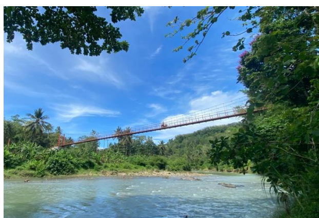
Figure 3. Condition of the bridge and school in Sukaluyu Village, Cikadu District, Cianjur Regency, Saturday (30/11/2024).
